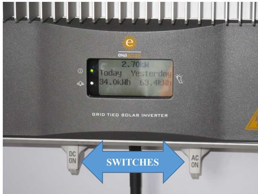
Figure 6: DC and AC Switches on Inverter
