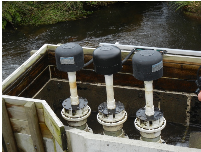
Figure 14: Turbines at NKNT
