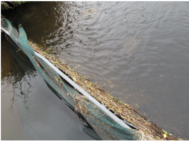
Figure 25: A Close Look at the Intake Congestion
