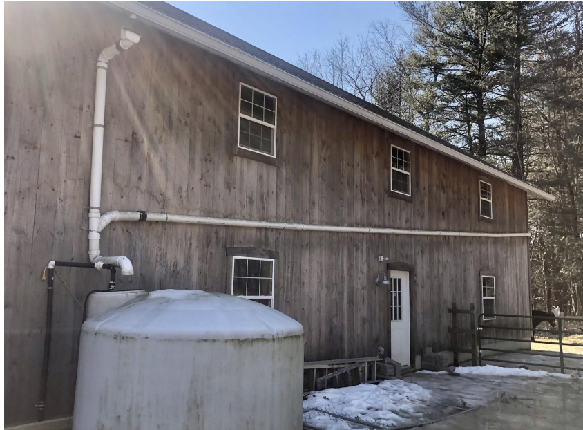
Figure 5: An example of a rainwater catchment system utilizing a roof and gutter system
