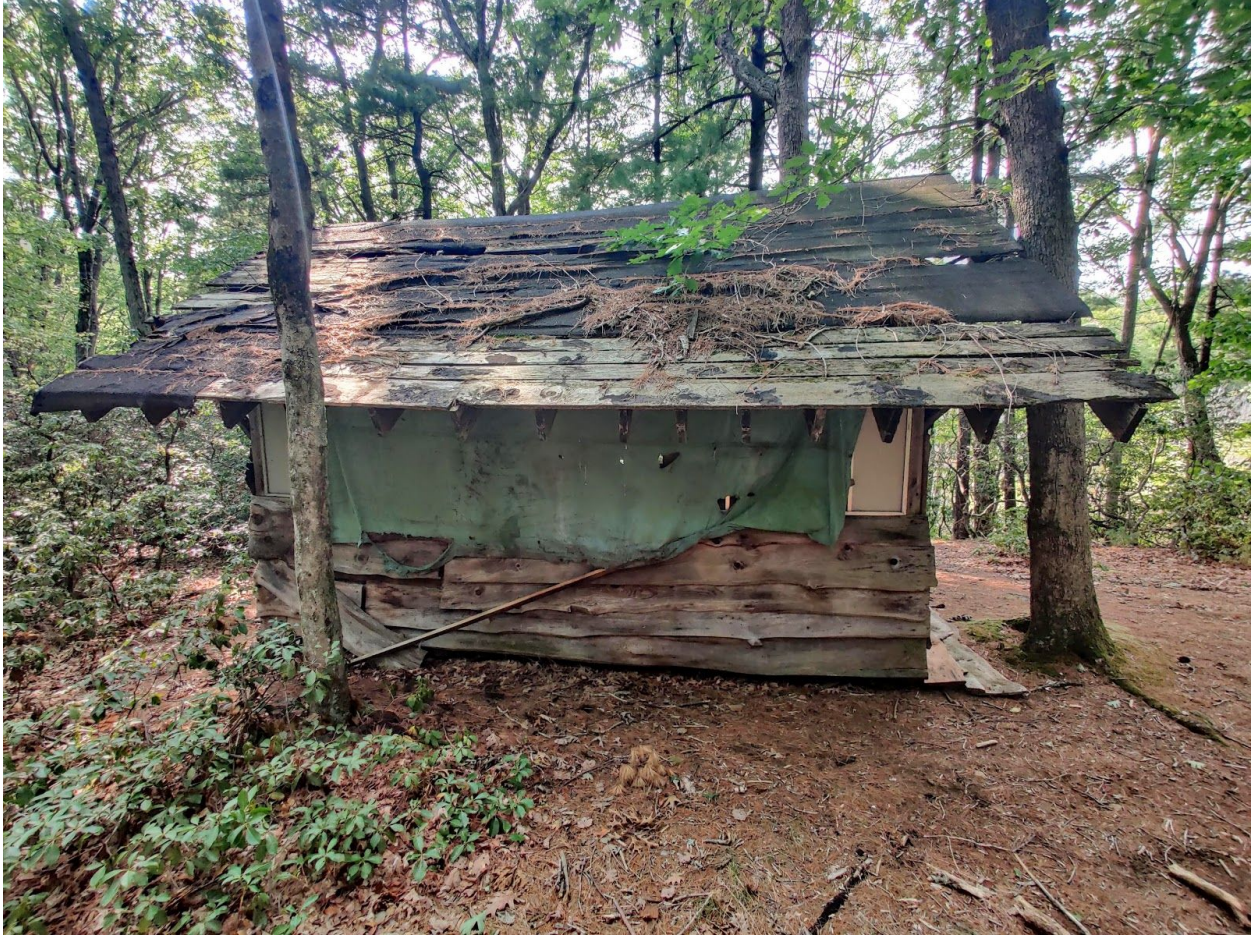
Figure D.3.4 - Heins Farm Cabin - This cabin, namesake for the Cabin Loop Trail on the Heins Farm property, is set to be torn down in the autumn of 2020, due to its poor condition and the use of hazardous materials in its construction (Dave Barnicle Interview, see appendix A).
