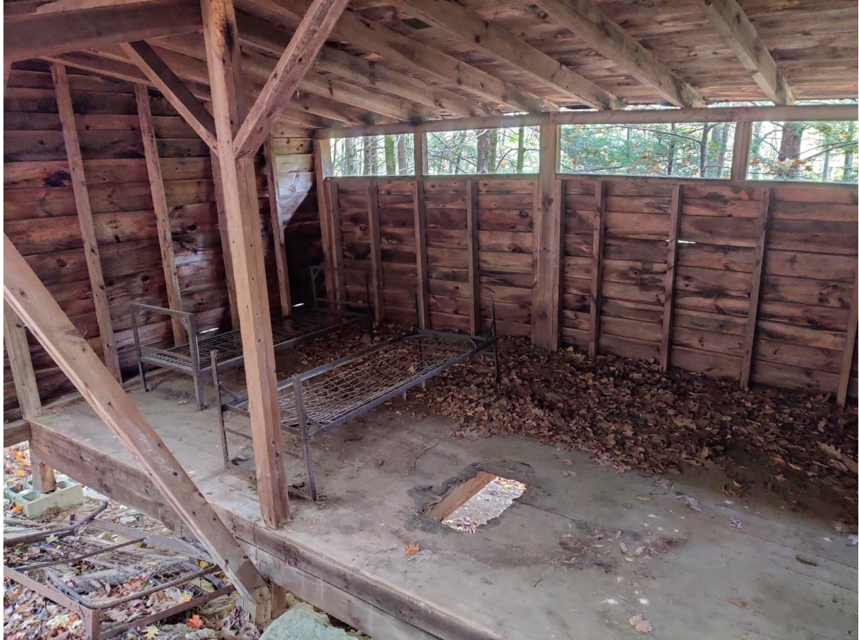
Figure D.3.3 - CRC Outbuilding (Interior) - Pictured above is a structure similar to that in figure 21, although not yet collapsed. As stated above, bed frames can be seen inside.
