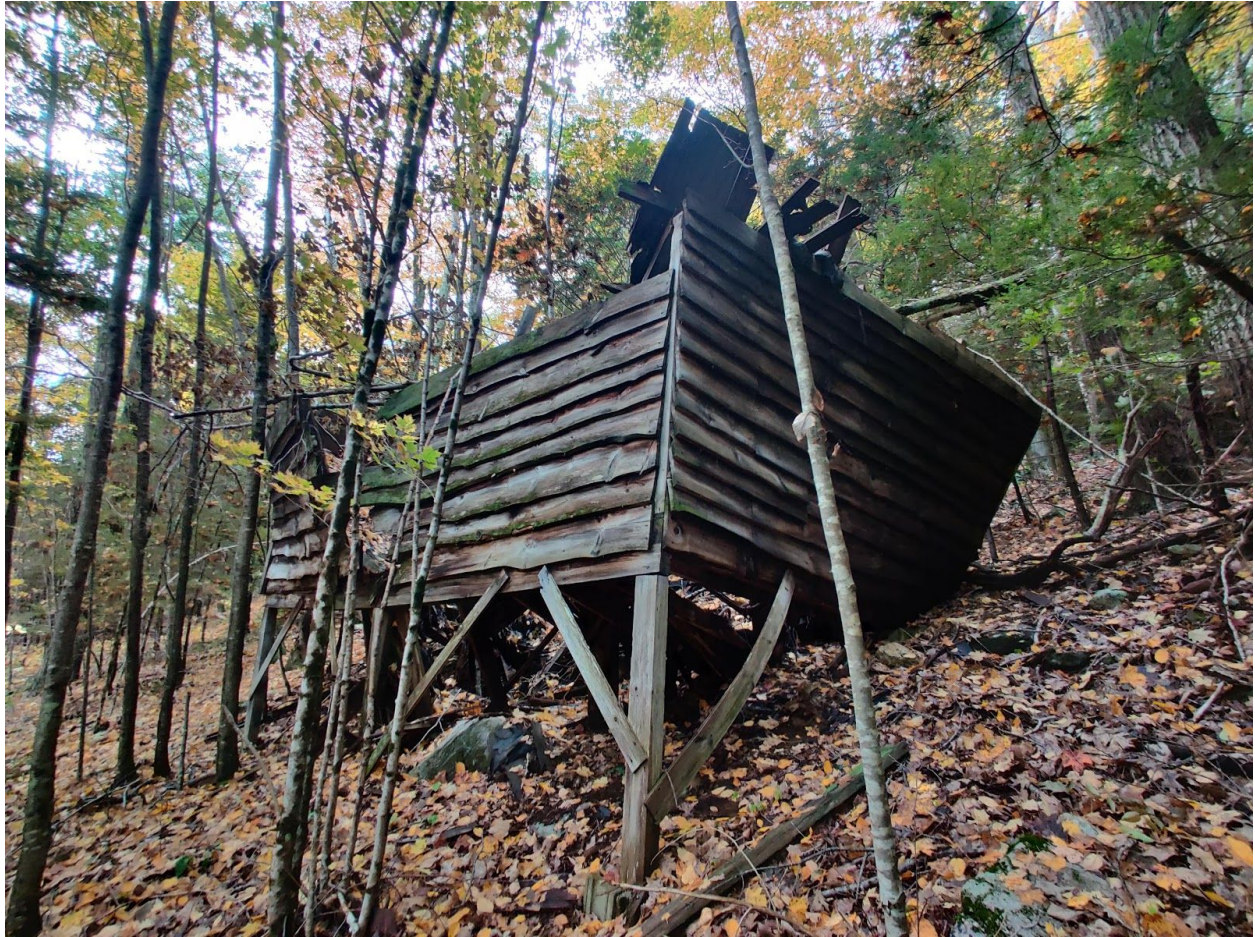
Figure D.3.2 - CRC Outbuilding (Exterior) - This structure is situated on a hill with another like it along with an outhouse. Although mostly collapsed, there are beds inside, signifying its use as sleeping quarters during the time of Camp Robinson Crusoe.
