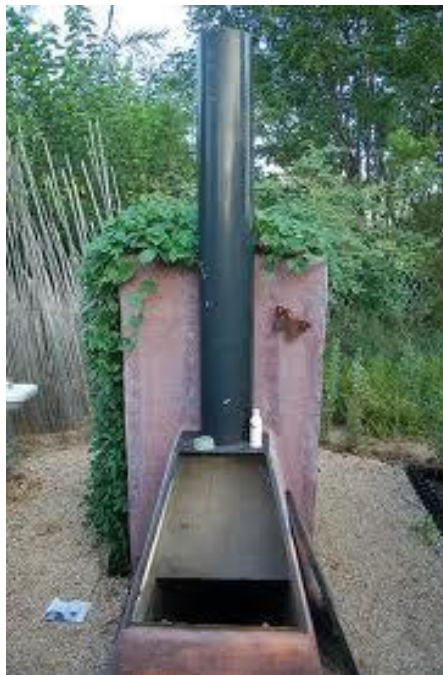
Figure 7: Dry sanitation Otji-Toilet system (Image by Boutin, 2011)
