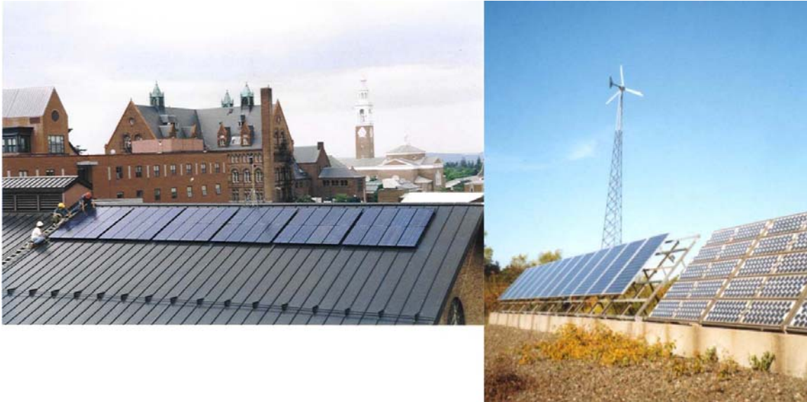
Figure 11: PV Installations - Left: UVM 48 , Right: Solar Now 49
