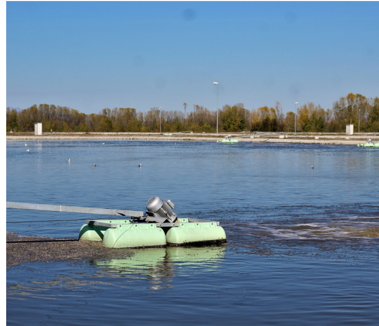
Picture of aerator from UKKO's facility in Korçë city
