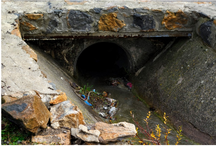
Open Drainage Pipe in Kamenicë.
