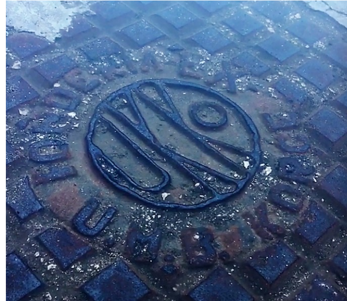
Picture of an UKKO manhole cover in Korçë city.
