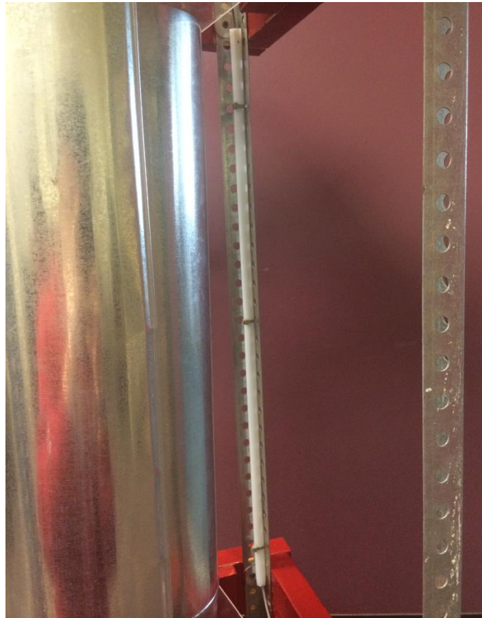
Figure 3-6: Safety Tubing for Power Cable from PV Module
