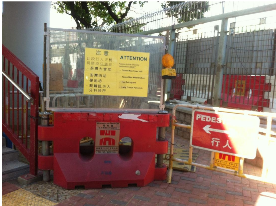
Figure 8: Exit indicators for a skywalk in Tsuen Wan due to ongoing construction
