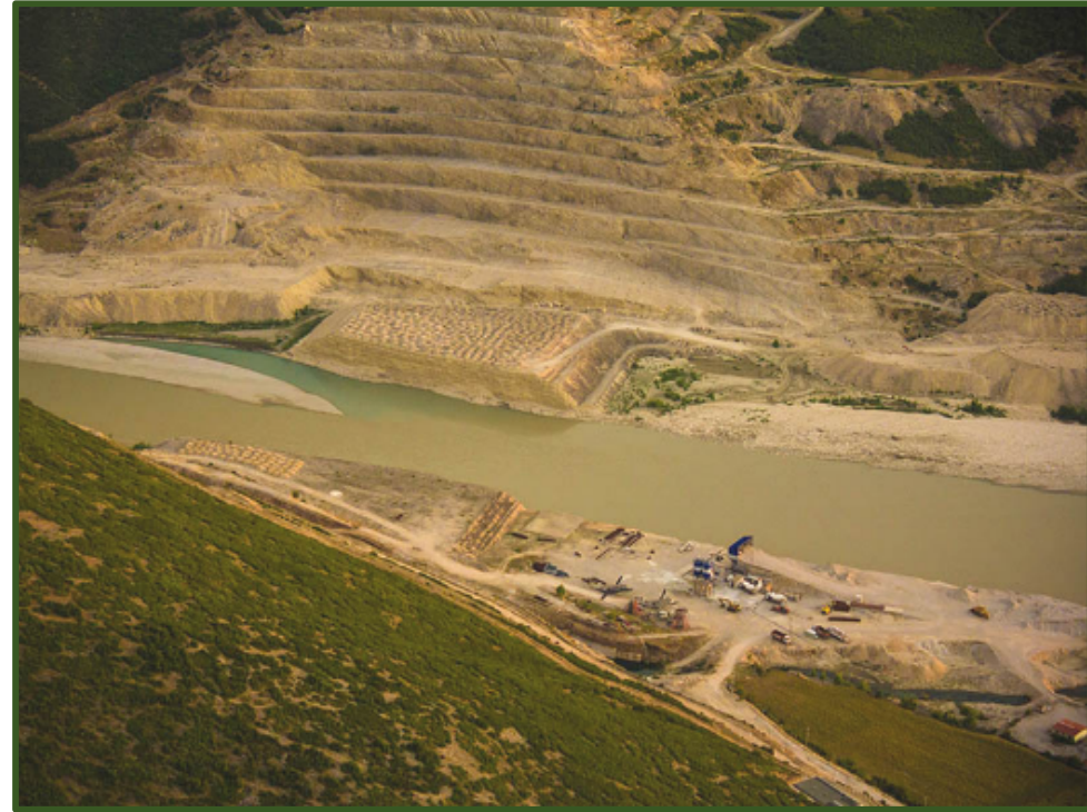
Figure 2.12: HPP Pressure in Vjosa Basin: Abandoned Works in Kalivaci, Vjosa River (MJEDISISOT.info/index.php/component/tags/tag/236-lumi-vjosa)
