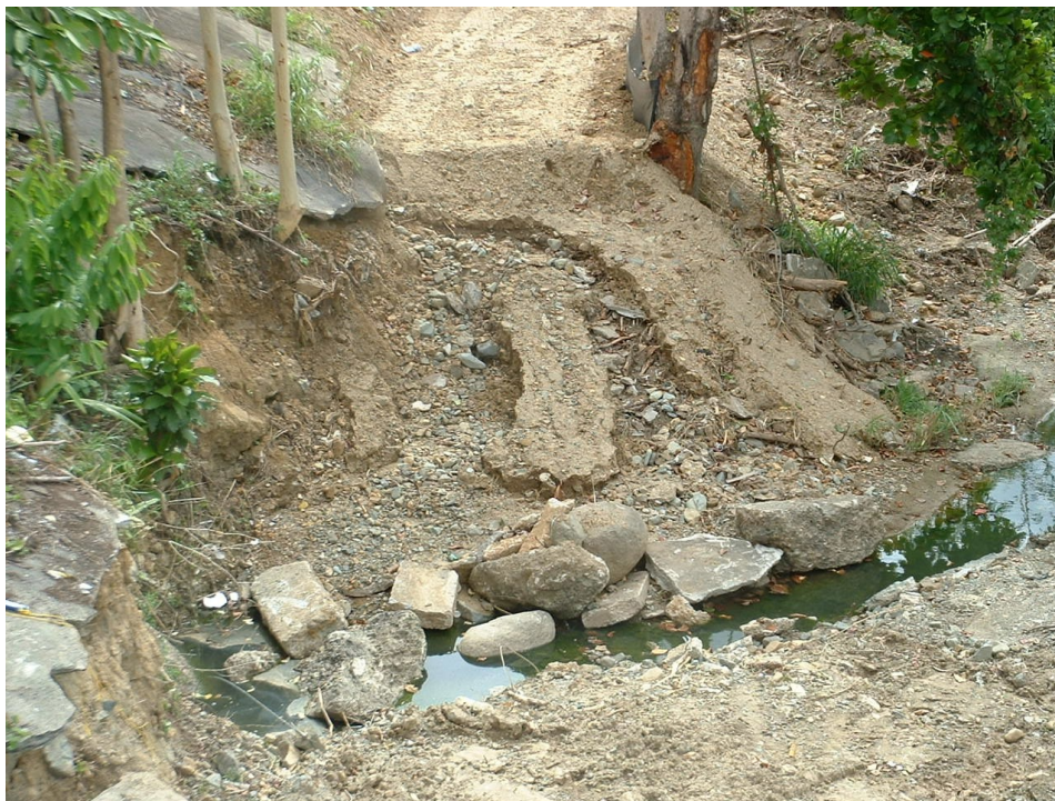
Figure 3: Example of gully erosion along the banks of the Caguitas River
